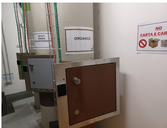
Fig. 4. Picture shows one of the four the drop-off points distributed in the terminal. The three doors, as well as the area, are accessible only to authorized personnel
