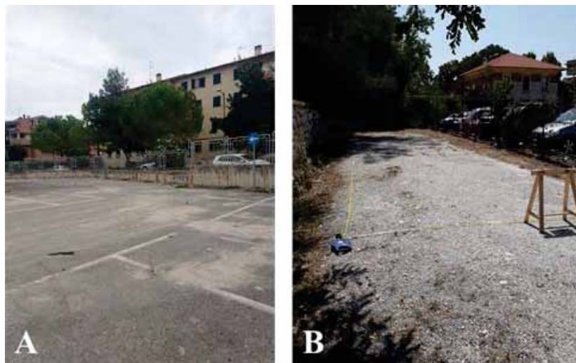
Fig. 3. Abandoned parking lots granted from the municipality of Ancona. Fig. 3A: First lot covered with a compact and undamaged asphalt layer; Fig. 3B: Second lot covered with deteriorated asphalt
