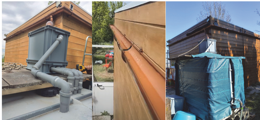
Fig. 3. Rainwater collection system installed at “Ai 300 Scalini”, Bologna. Source: Pictures taken by the authors
